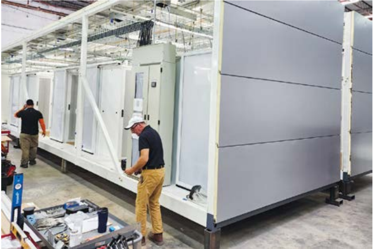
Assembly of an iM Data Centers stand-alone enterprise-class data center in Fort Lauderdale.
