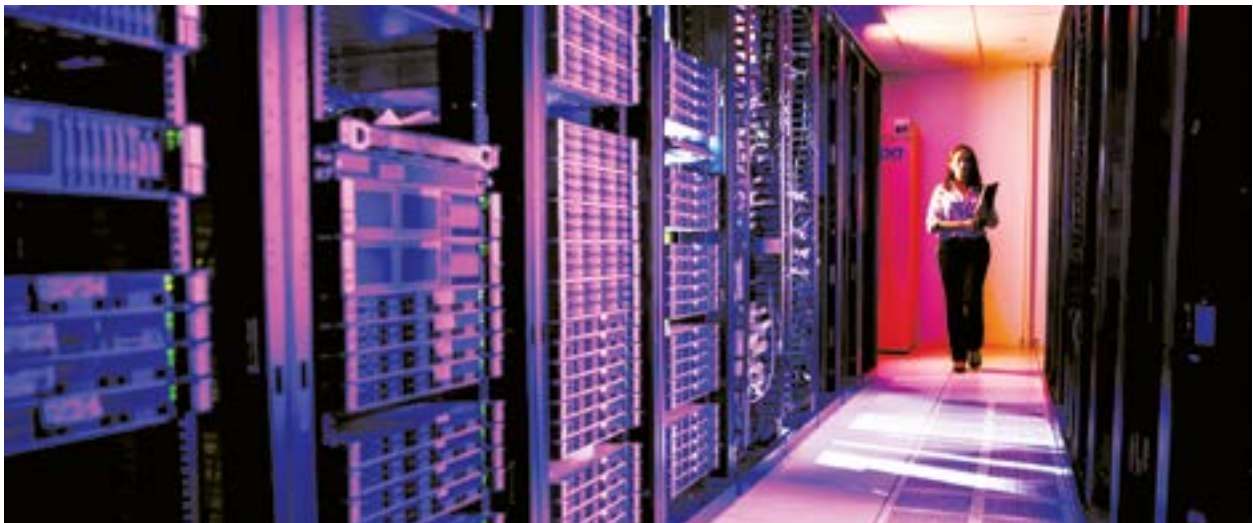
Hotwire Communications server room in Fort Lauderdale
